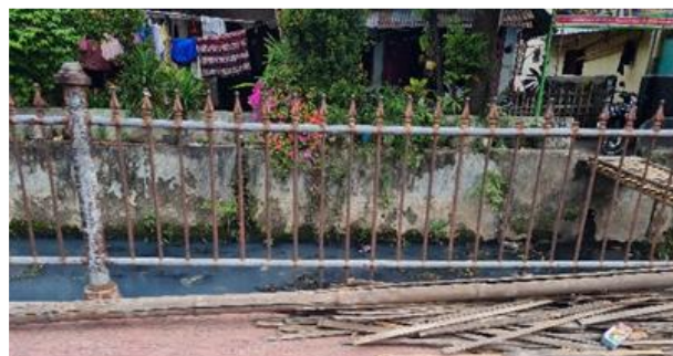
Figure 12. Condition of Jl. Jagasatru Sidewalk
