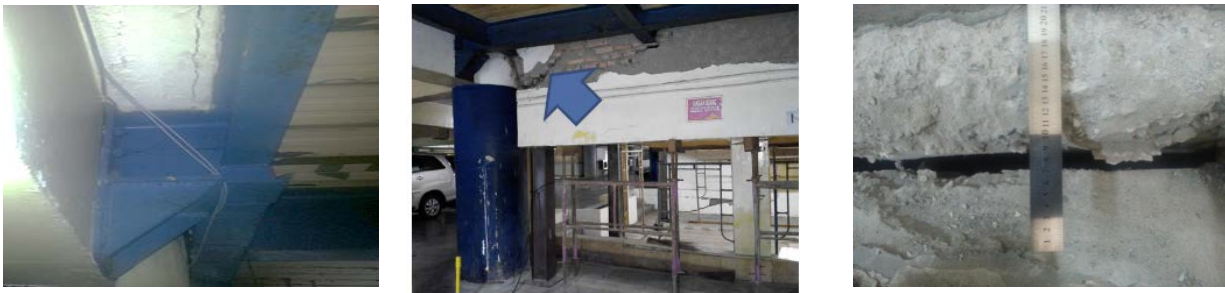
Figure 2. Damage to the upper structure
