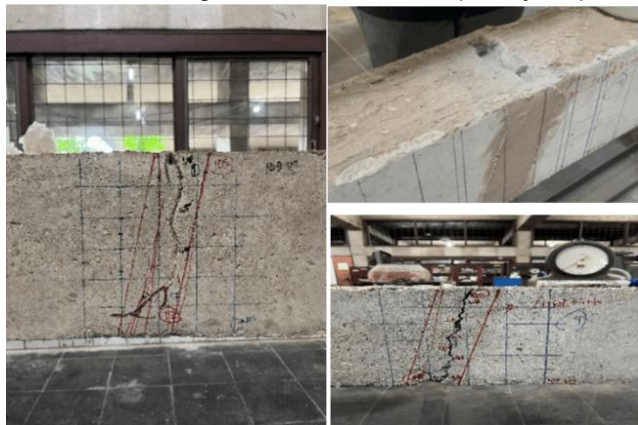
Figure 9. Chiseling around the cracked area of the beam specimen
